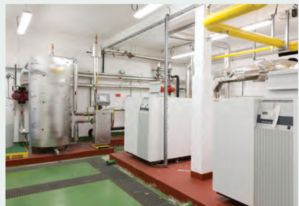
Engie boiler plant at Ris Orangis (91)
